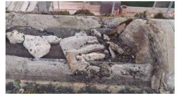
Bat droppings under ridge tile
