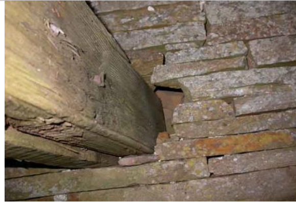
Internal gaps near loft beam
