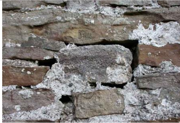
Missing stone mortar
